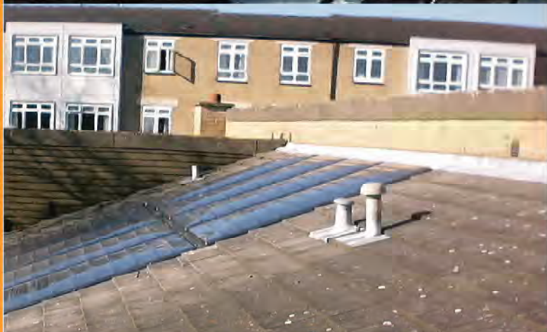
Installed by Imagination Solar's accredited agent, Southern Solar
